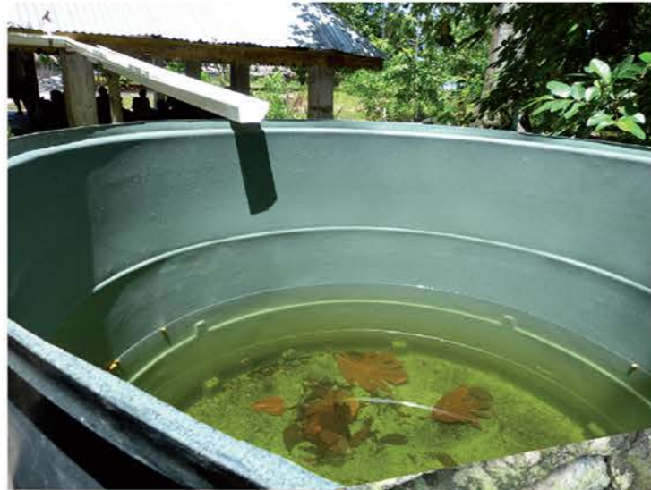
Unprotected rainwater tank, Carlo Iacovino, SPREP 2013
